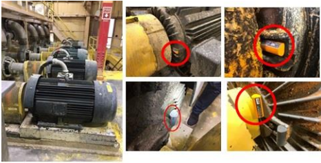
Figure 4. Deployment of wireless vibration and temperature sensors in manufacturing plant.
