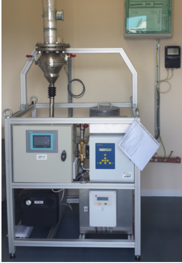
Figure 1. Ventilation Gas Monitor (VGM) (Perrin, 2018).
